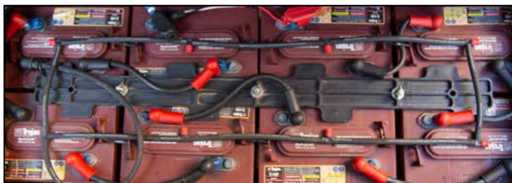
Automatic Battery Watering System
